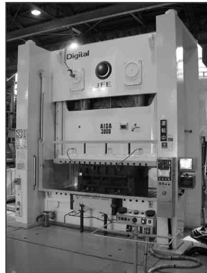
Photo 1 Servo press machine installed JIM-Form technology
